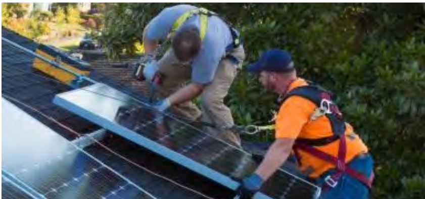
Typical Photovoltaic Installation
